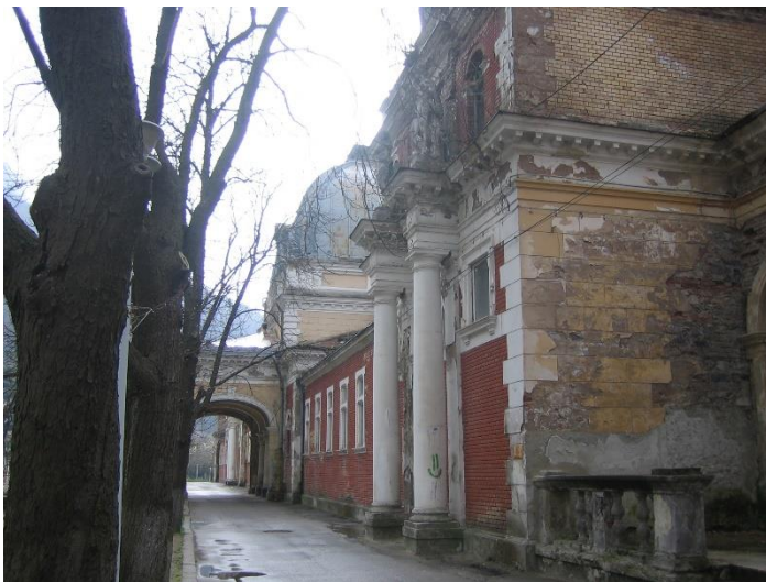
Figure 12: Devasted spa hall in the old spa ensemble of Băile Herculane. Photo: JORDAN 2011.
